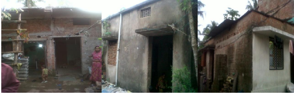
Photo 4. Makeshift arrangements by beneficiaries in partly constructed DU's
