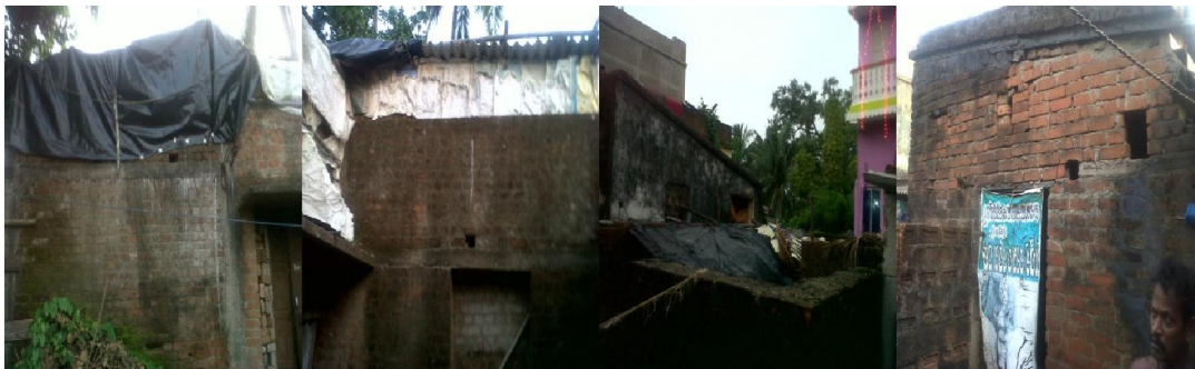
Photo 3. Roof covered by polythene sheet or asbestosin partly constructed DU's
