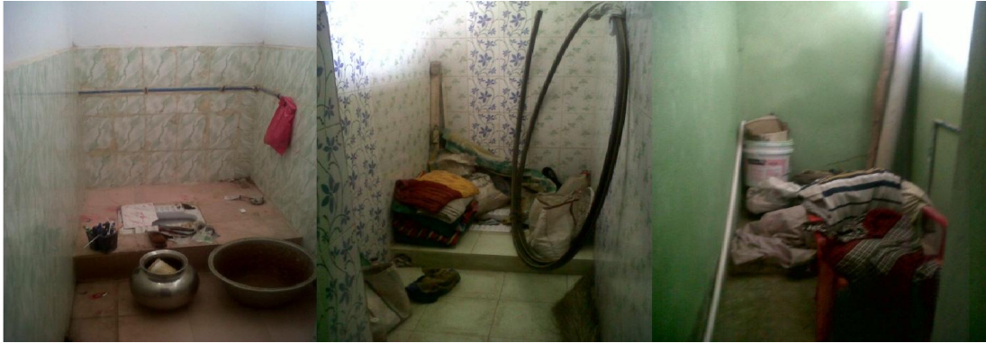
Photo 7. Toilets in completed DU's used as storerooms
