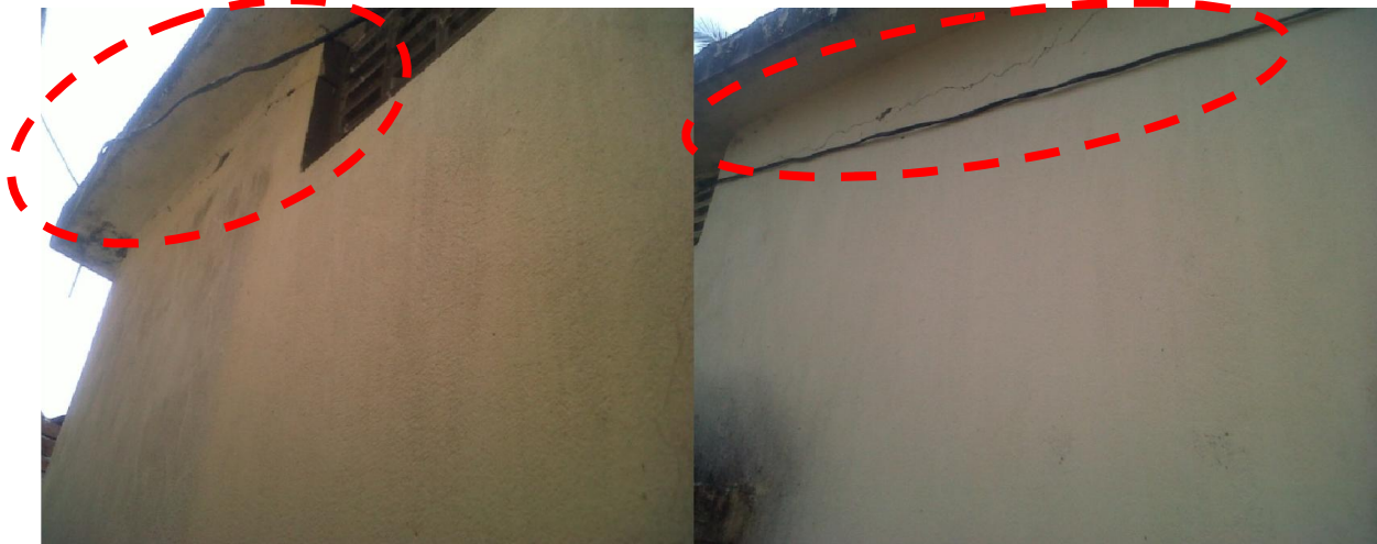
Photo 9. Cracks in roofs of completed DU's
